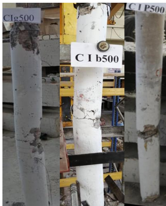
Fig.8. Crack pattern and Failure Mode of Tested Composite Columns
